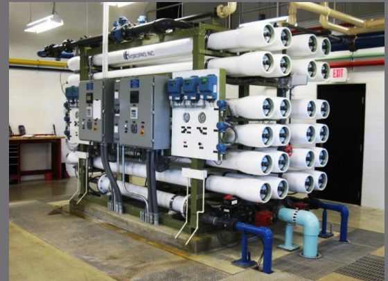
Figure 1. Image of reverse osmosis system at the municipal water plant
